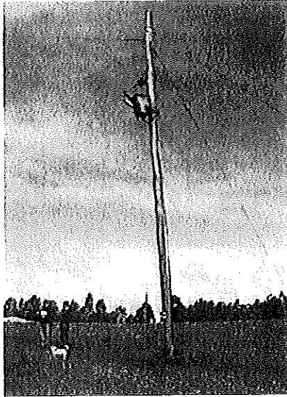
Plate 6: The 35kV transformer installed by the landowner located on the western boundary of the amendment site, approximately 315m from Brockman Highway.
