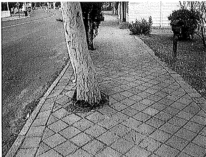
Brick paving footpaths are uneven as a result of tree root damage.
